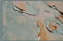
Peeling & Flaking of paint
